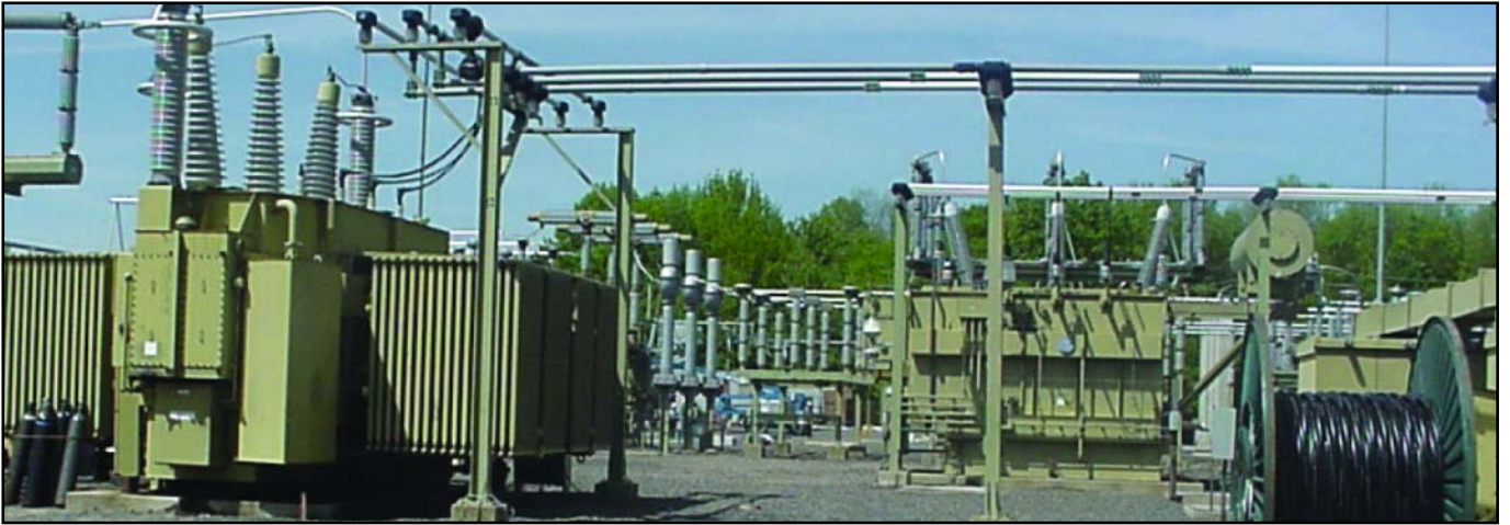
Jackson Road Substation - 45MVA - 230/13kV, Transformers T3, T4
