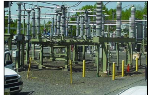
Jackson Road Substation 230kV Pothead Termination
