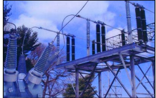
Athenia Switching Station 230kV GCB 71H Load, Side Disconnect View
