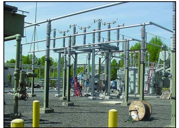
Jackson Road Substation- 230kV Disc. Switch
