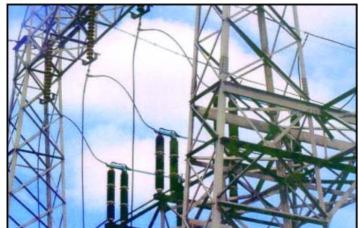
Athenia Switching Station 230kV Switch 70J60 Tower
